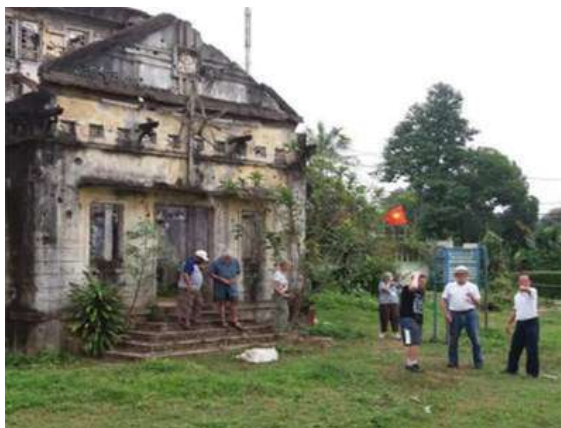
Long Hung Church, Dong Ha. One of only two structures in Quang Tri Province by the end of the war. Destroyed, but still standing,
